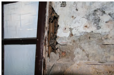
●禮拜堂木窗及牆面損壞
