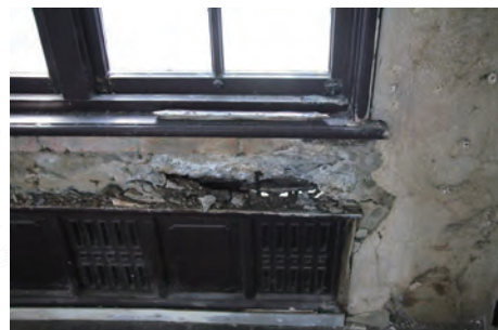
●禮拜堂木窗及牆面損壞
